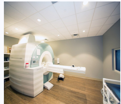
RF Shielded MR room
